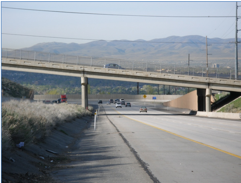
Figure 1 Presence of Steep Grades
